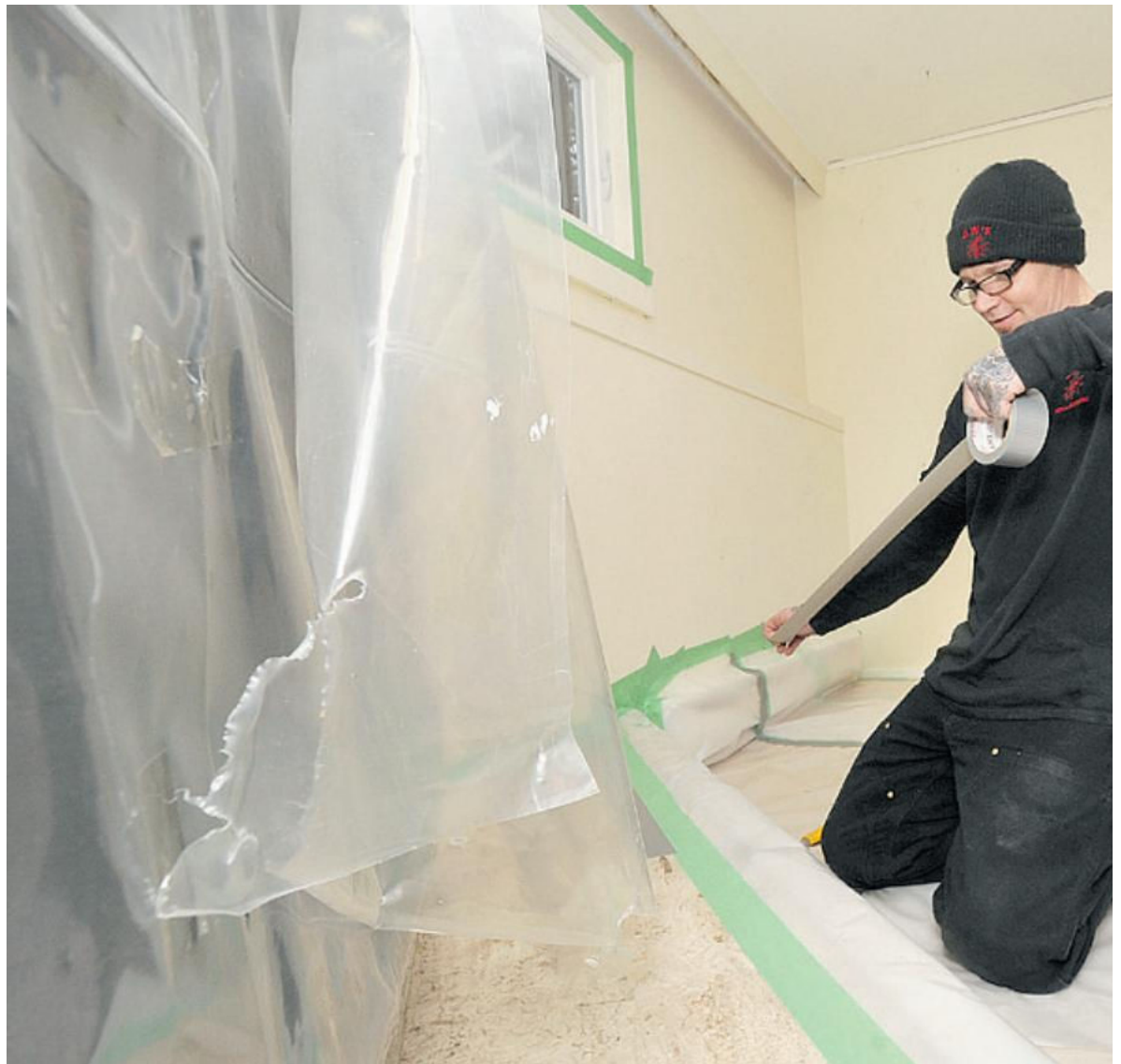
Wayne Lei 4W's Demo project manager Ralph Kettle follows all the guidelines and regulations when removing asbestos.
