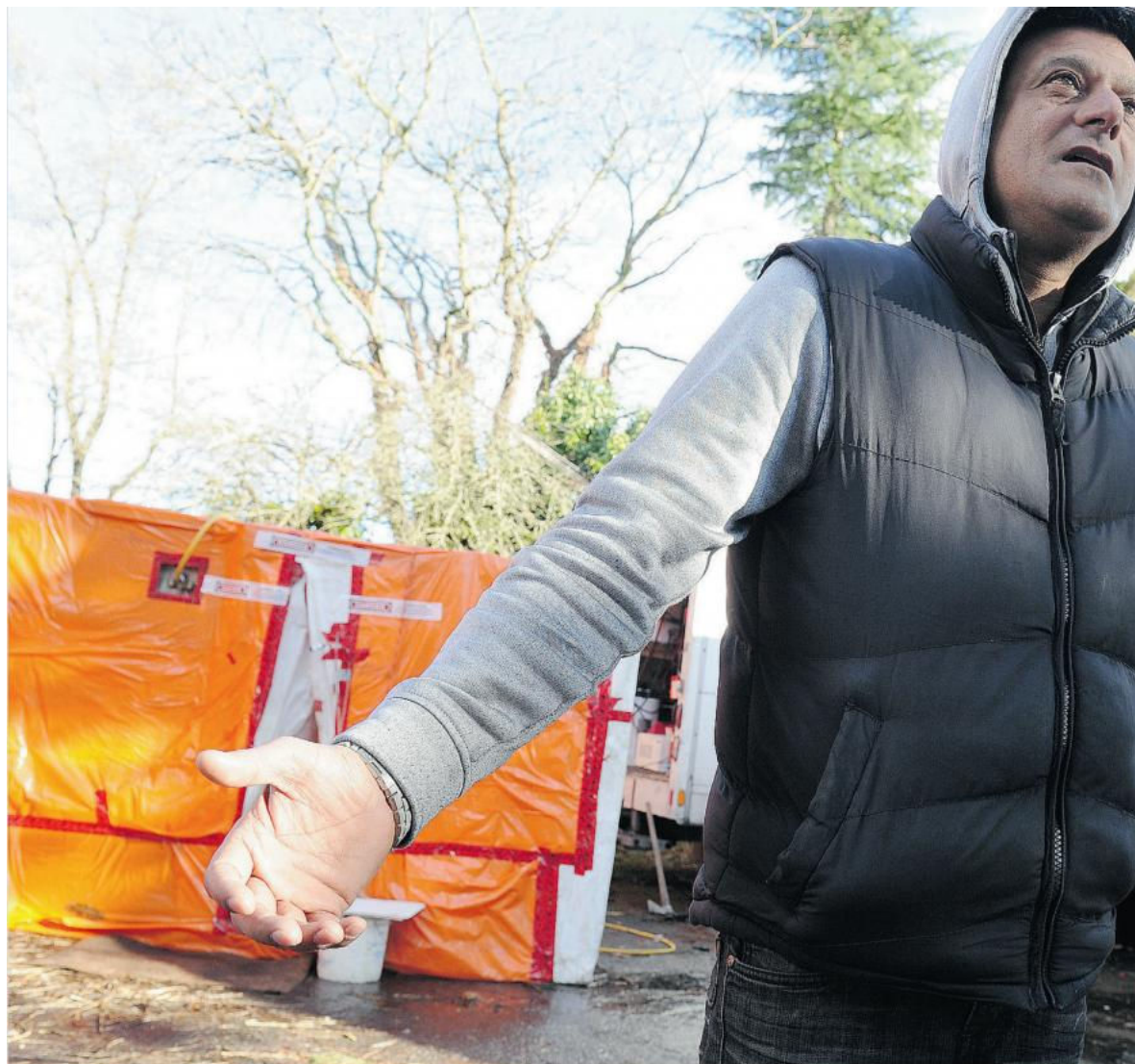
Mike Singh and his companies have been issued hundreds of orders for breaking rules in removing asbestos and they have also been fined. Singh says he has not broken the rules and Photograph by: Jenele Schneider, PNG, Vancouver Sun
